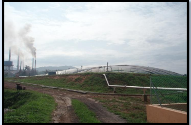
Completed cover with captured gas showing pipe leading to the flare
