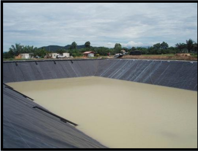
Base and slopes lined with 1.5mm thk. HDPE Liner
