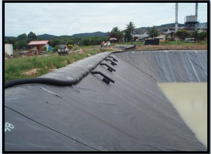
Gas collection pipe for bio-gas collection.
