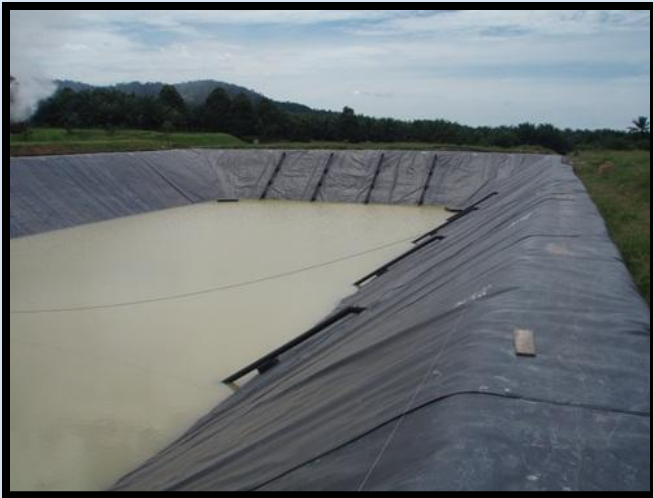
View showing influent pipes; far end and on slope desludging pipes.
